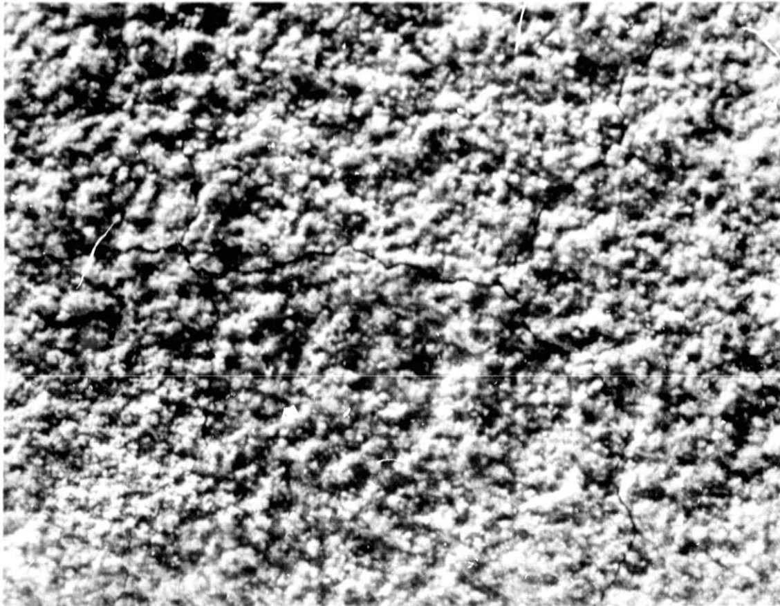
Figure 33 Radial (Mud Flat) Cracks – Thermal Fatigue Test No. 1 Baseline Seal System (77-441-0995-L)
