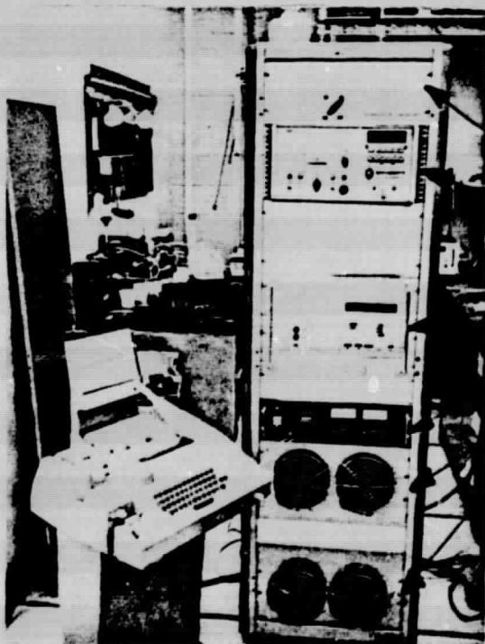
Figure 2. Front view of CFD control rack and Teletype. Equipment in the rack from the top is:
