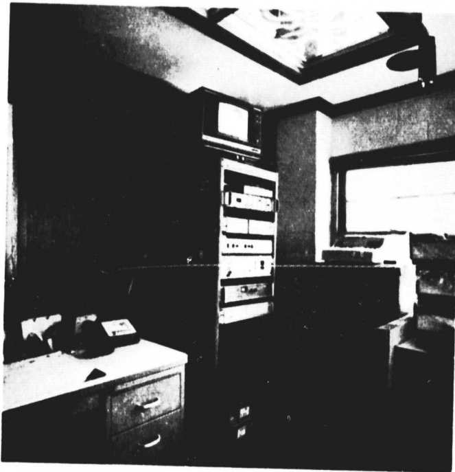
Figure 6-10. C-Band TVRO Equipment Installation
