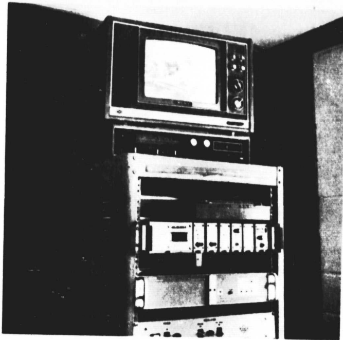
Figure 6-9. C-Band TVRO Equipment Receiver and Monitor
