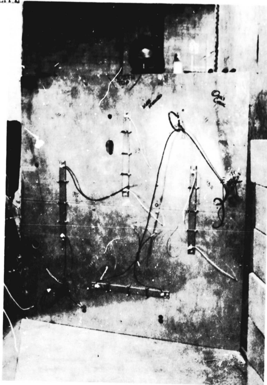
Figure 4-26. Reflux Boiler Aluminum Panel with Guard Heaters
