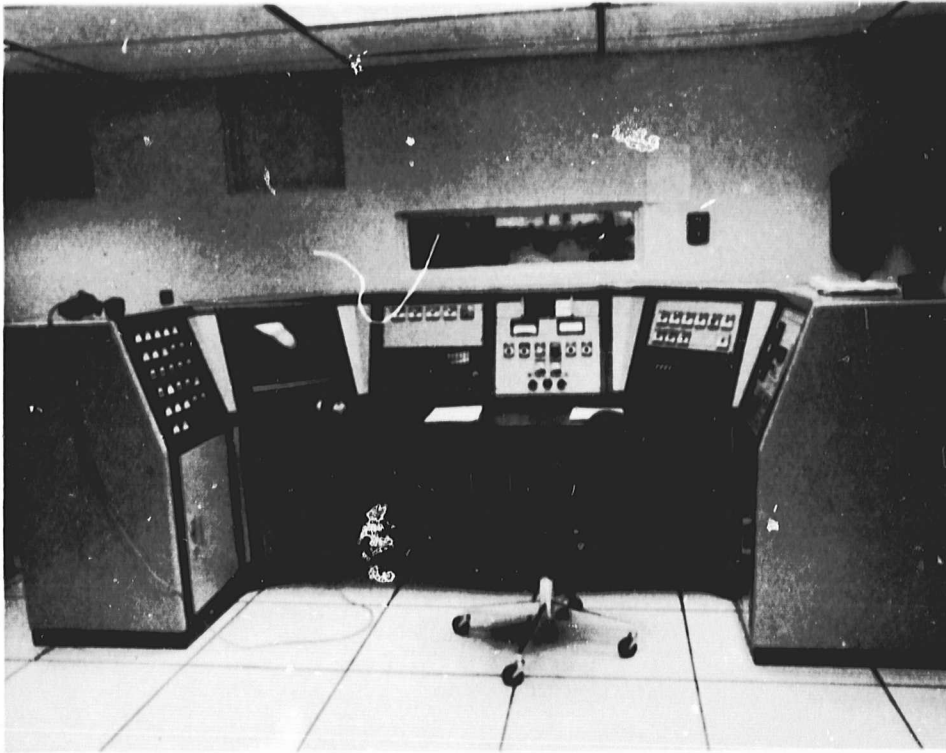
Operating Room of MTI Stirling Engine Test Cell
