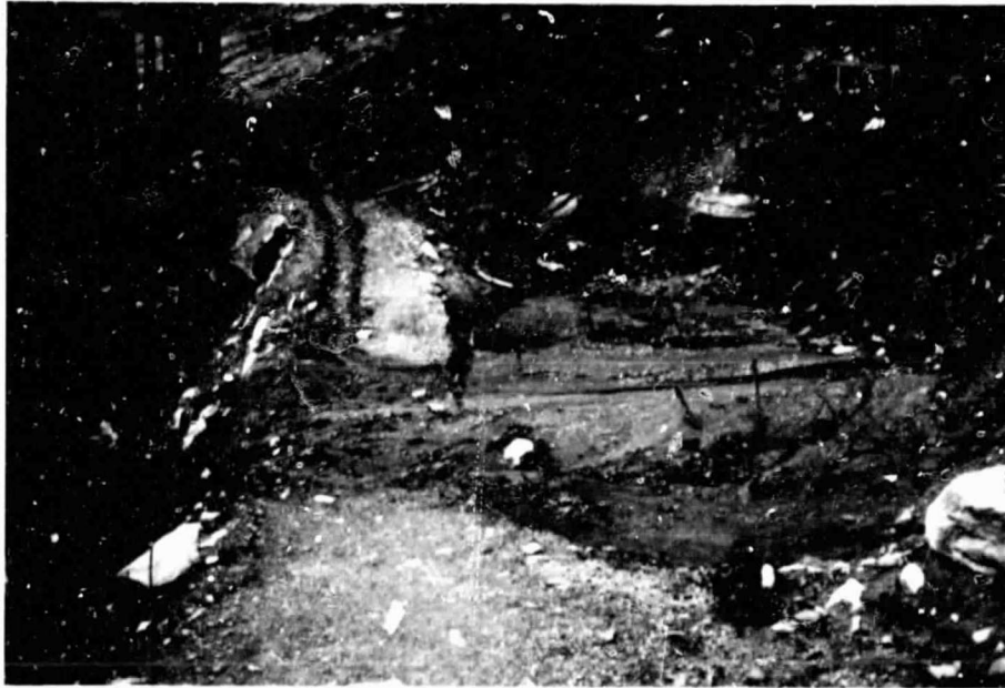
Figure 11. A caterpillar-constructed debris basin placed to intercept large volumes of silt and debris. Original depth of this basin was 4\frac{1}{2} feet.
