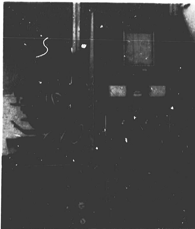
(c) Control Panel
