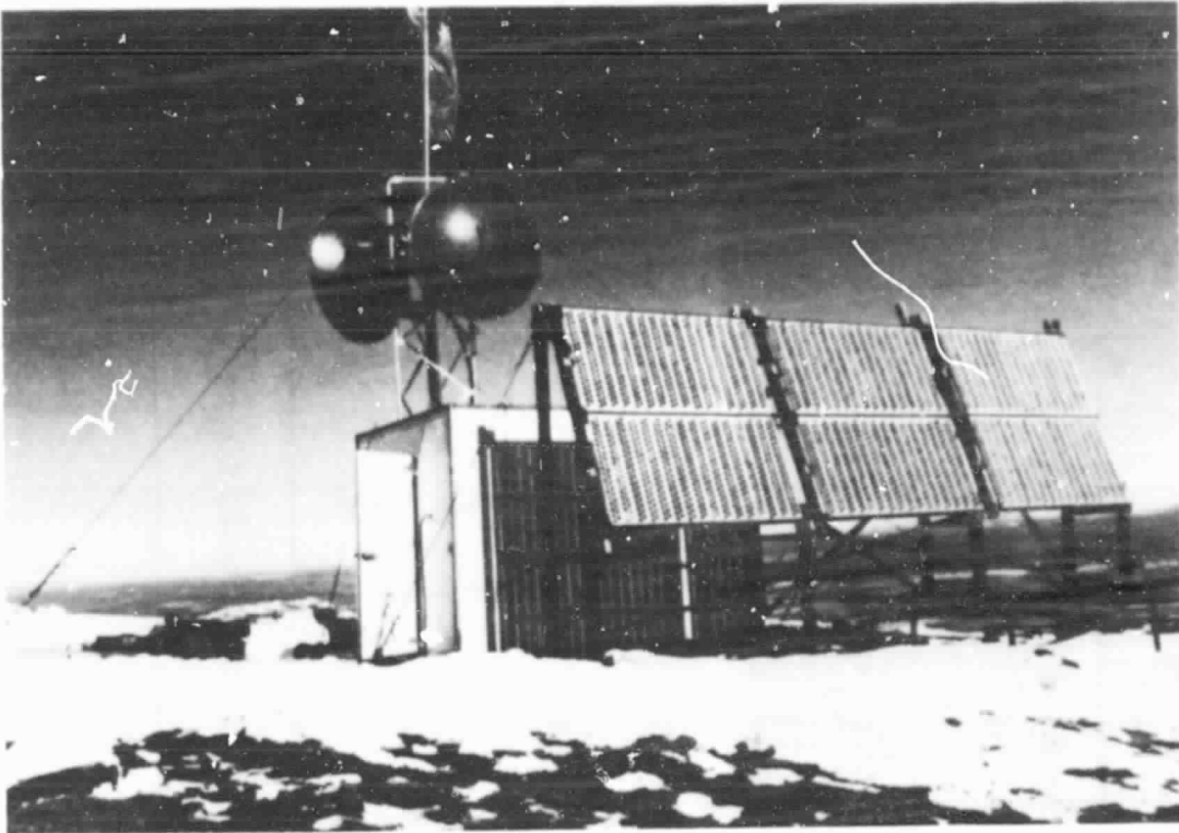
Figure 1. Microwave Repeater Station in Alaska (Courtesy of Spectrolab, Inc.)
