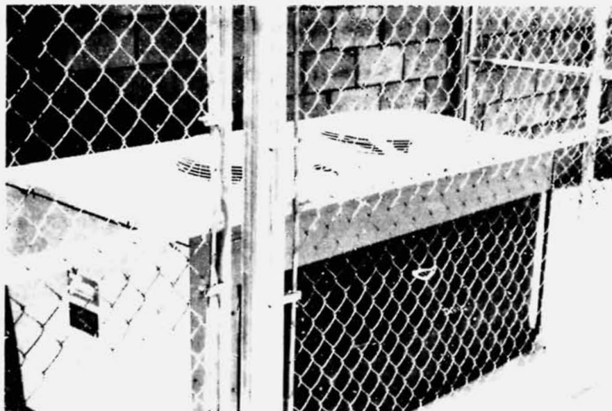
Figure 4 - External water chiller for regulating cooling water temperature.
