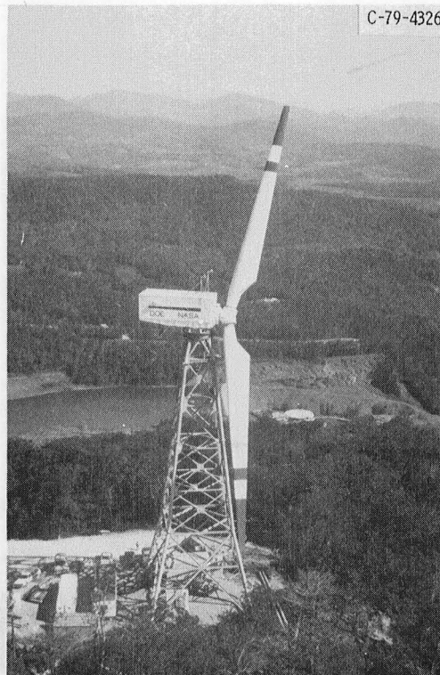
Figure 4. - MOD-1 experimental wind turbine.
