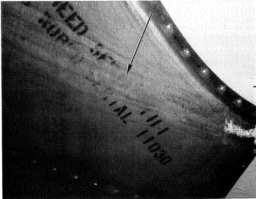
Figure B-5. - TWA left-hand aft engine fairing - Skydrol attack on vapor barrier
