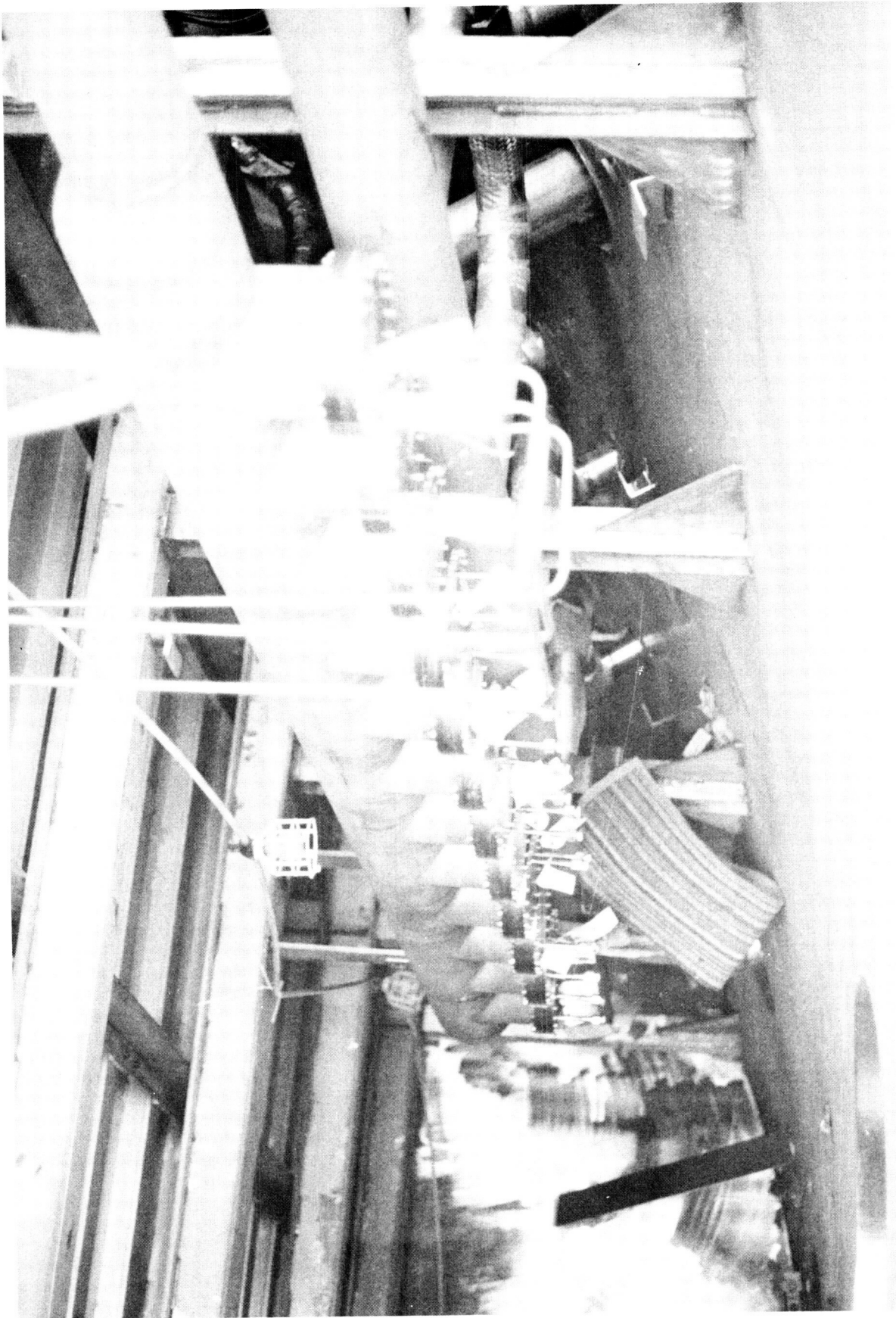
Figure 8. Discharge manifold vessel
