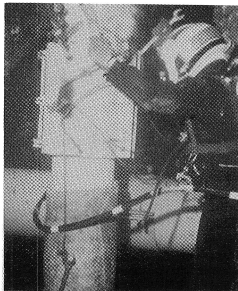
Diver Using an Impact Wrench to Tighten Bolts on a Riser Clamp. Note Use of Legs as Attachment Point
