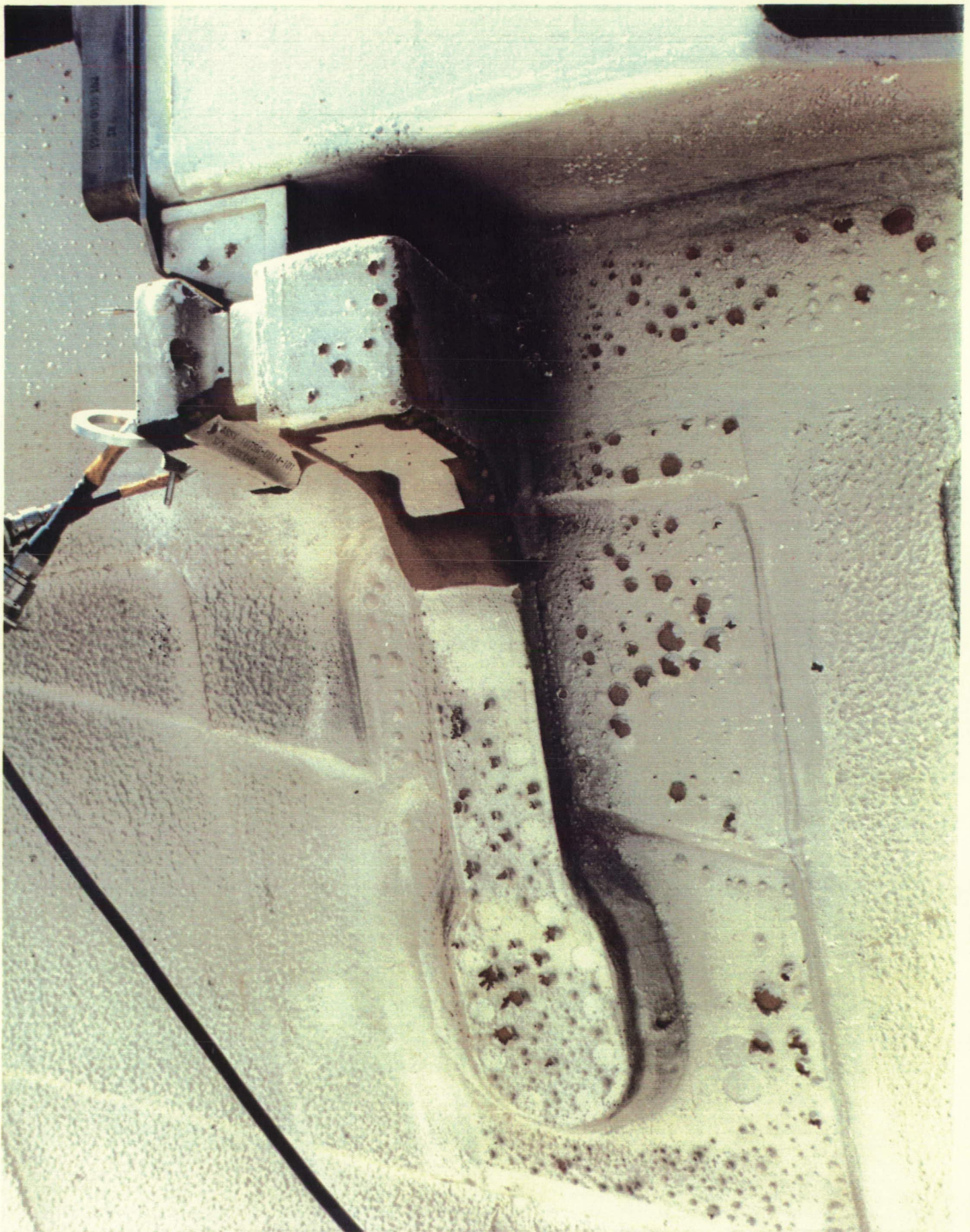
Localized areas of Hypalon paint blistered with some layers of MSA-2 adhering to the paint
