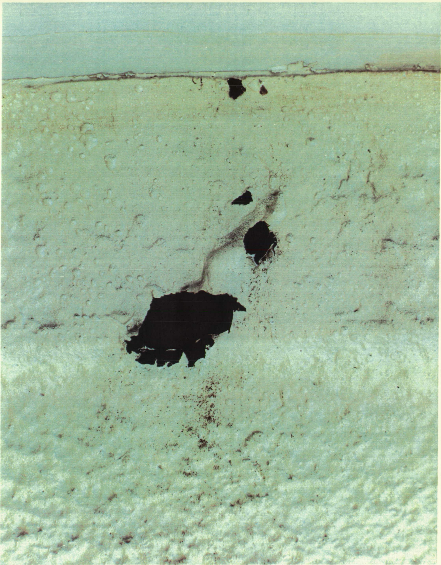
Layers of MSA-2 adhering to Hypalon paint blisters increases the mass of the paint chips and causes tile damage
