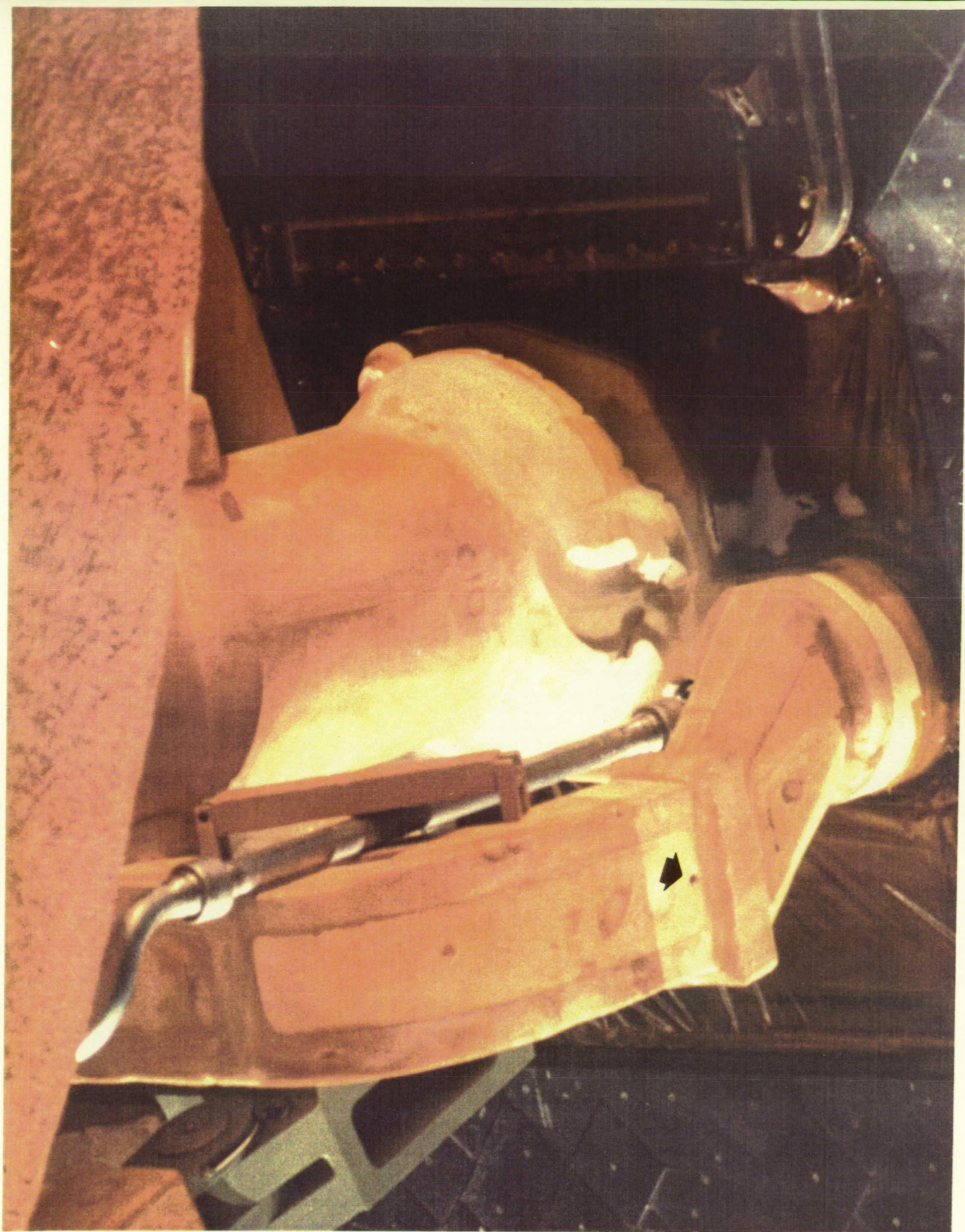
Normal appearance of ice/frost on the purge vents and aft side of the LO2 ET/ORB umbilical. Cable tray vent hole is clear.
