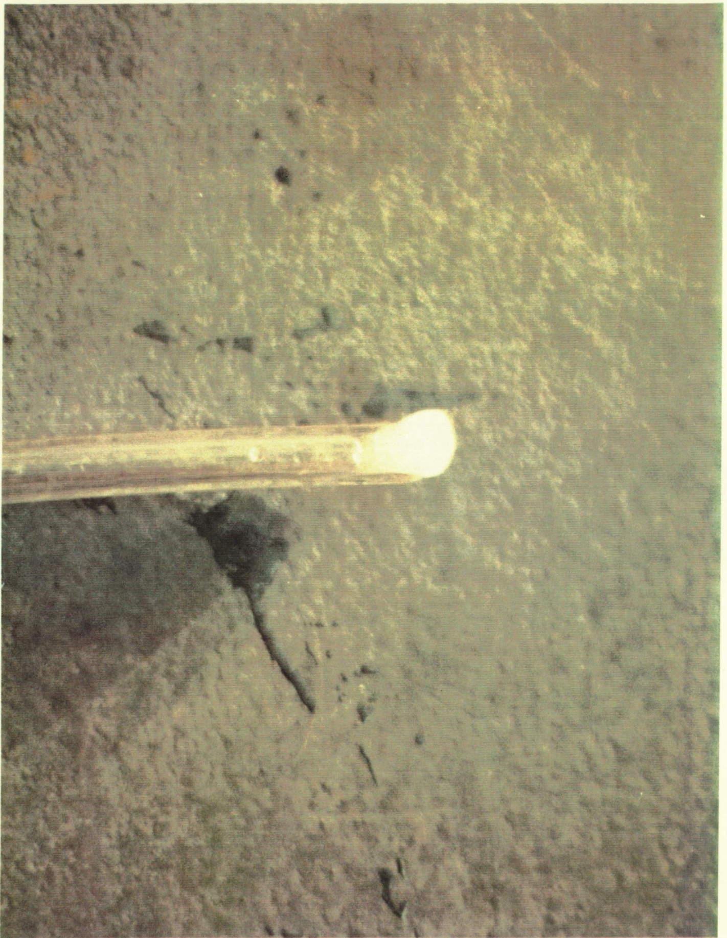
The hydrogen detection system tygon tubing drooped and became plugged when ice formed on top of the LH2 ET/ORB umbilical
