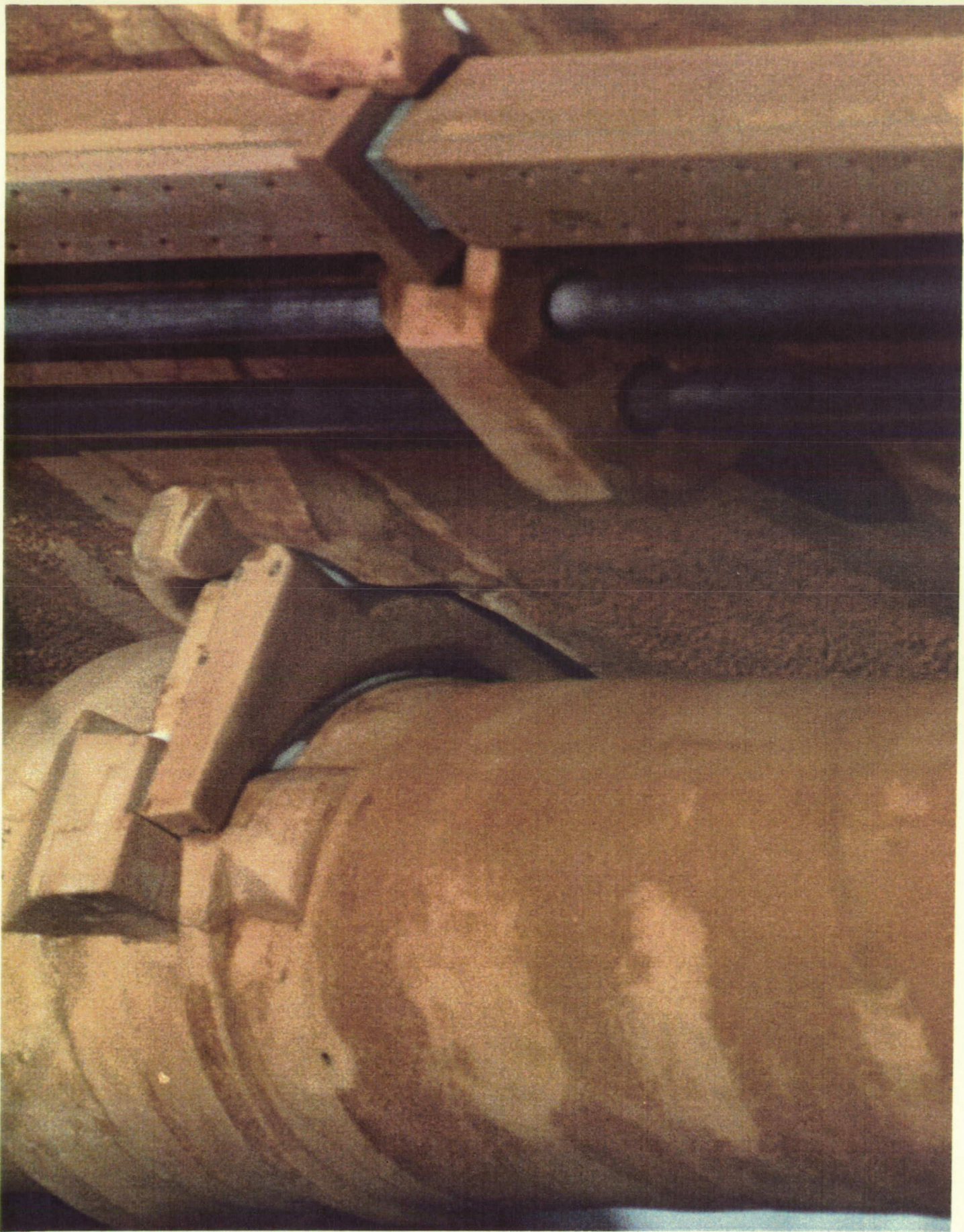
Typical accumulation of ice/frost in the L02 feedline support bracket. Note frost spot along aft side of ice/frost ramp.
