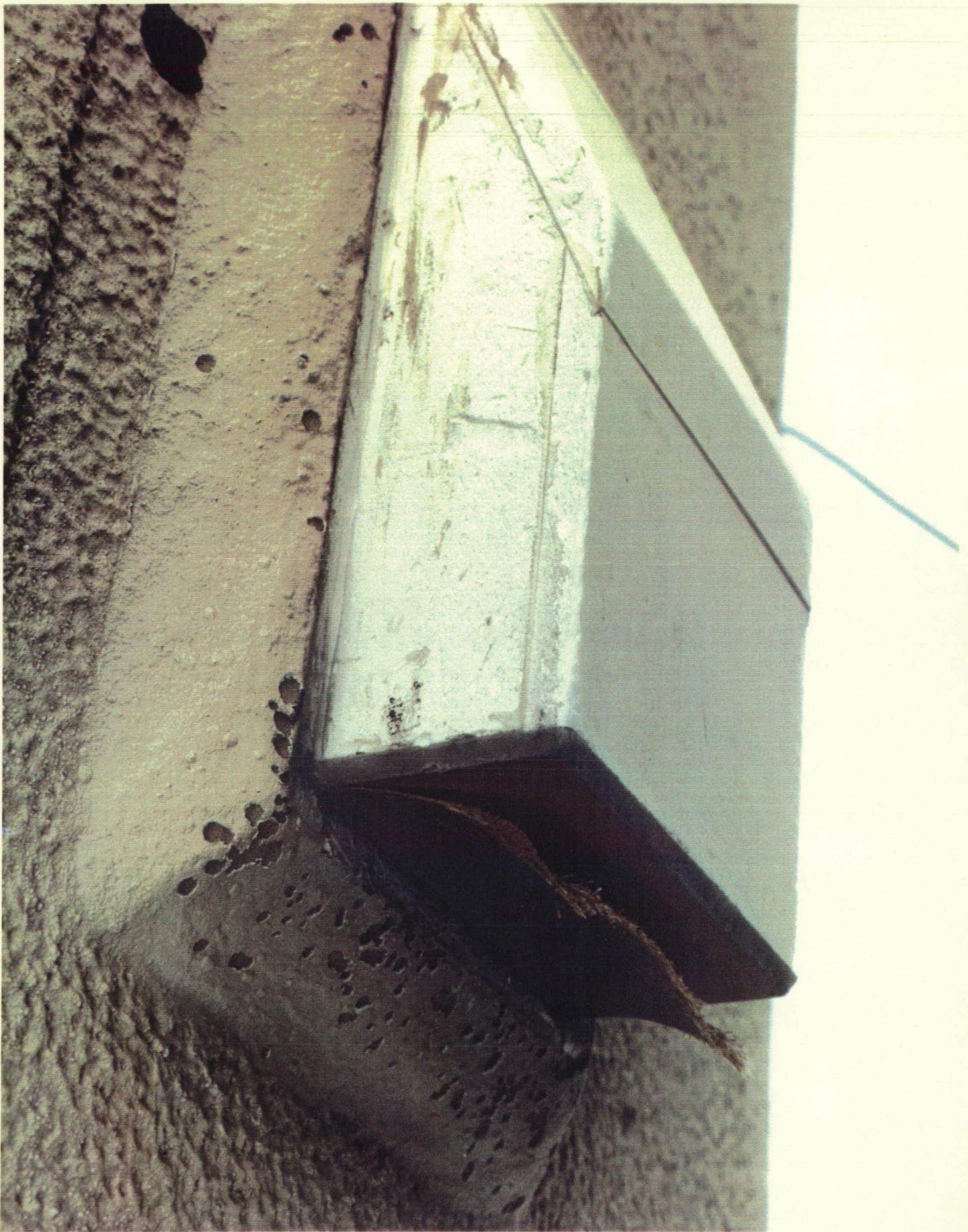
The phenolic plate on the -Z RSS antenna had some delaminated layers
