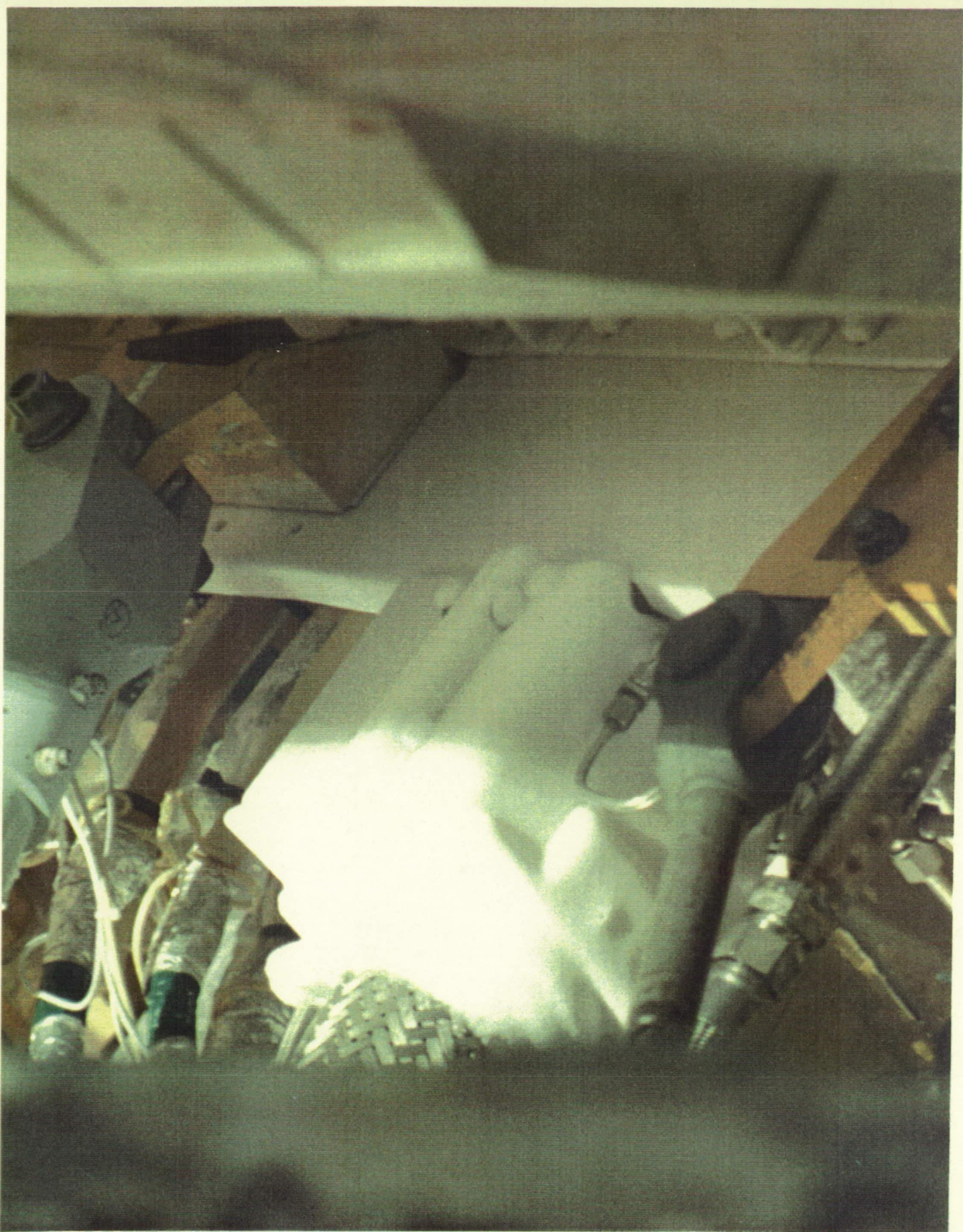
Ice/frost typically covers the 1-1/2 inch high point bleed QD purge shroud
