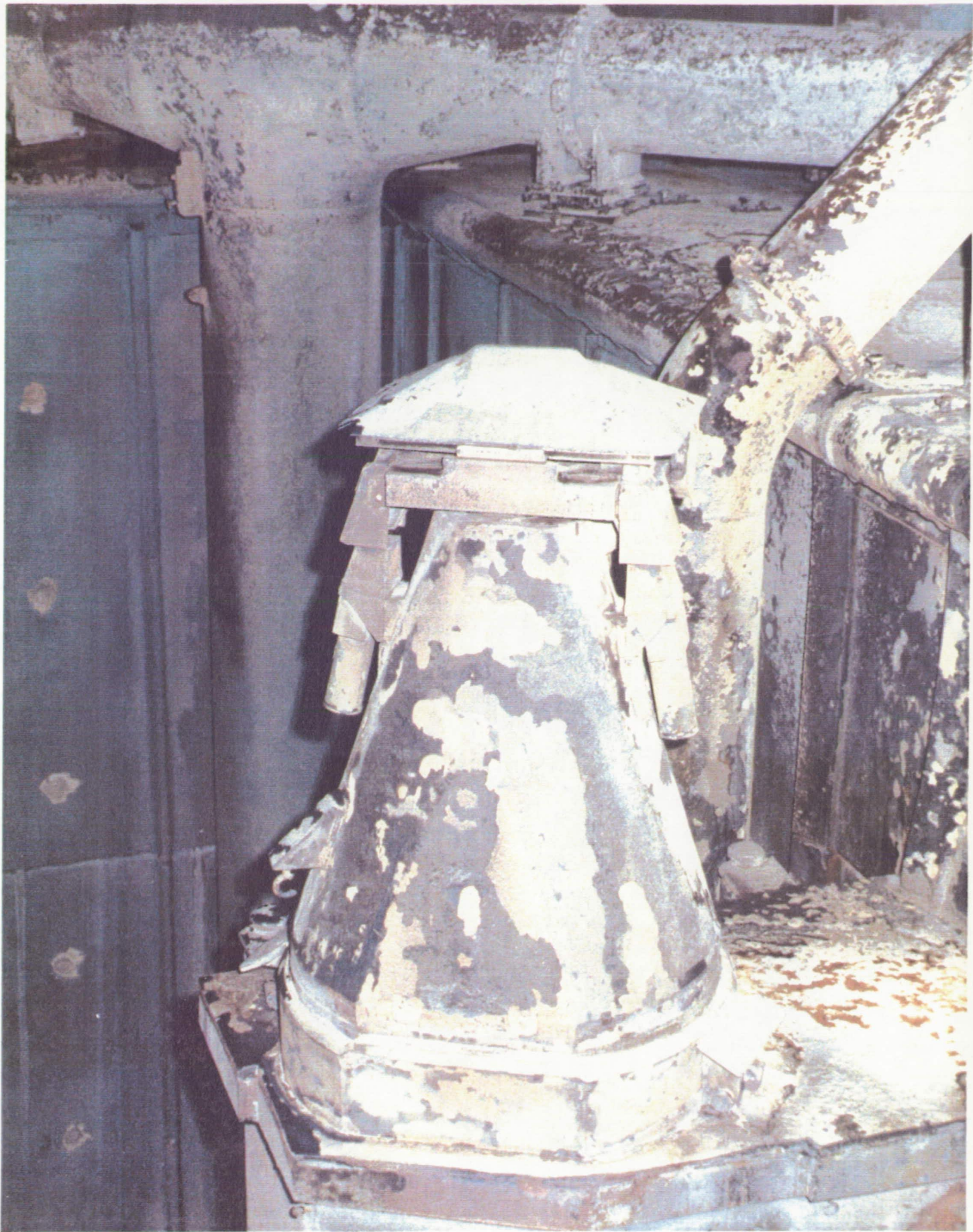
Typical SRB plume erosion on north holddown posts. All doghouse blast covers had closed properly.
