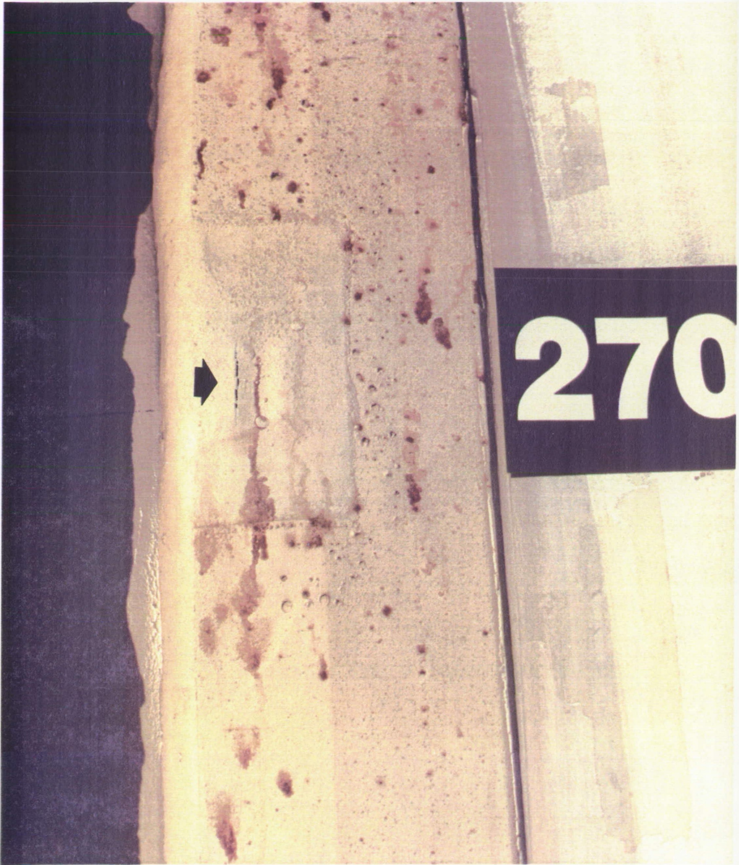
A 2.6-inch crack occurred in the K5NA closeout on the left aft field joint trunnion
