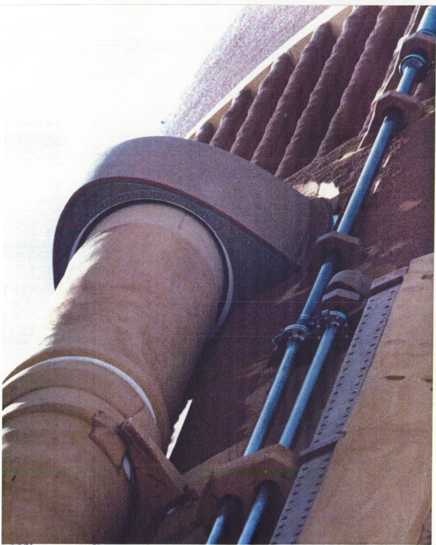
Ice/frost accumulations in the L2 feedline upper bellows and support brackets were typical
