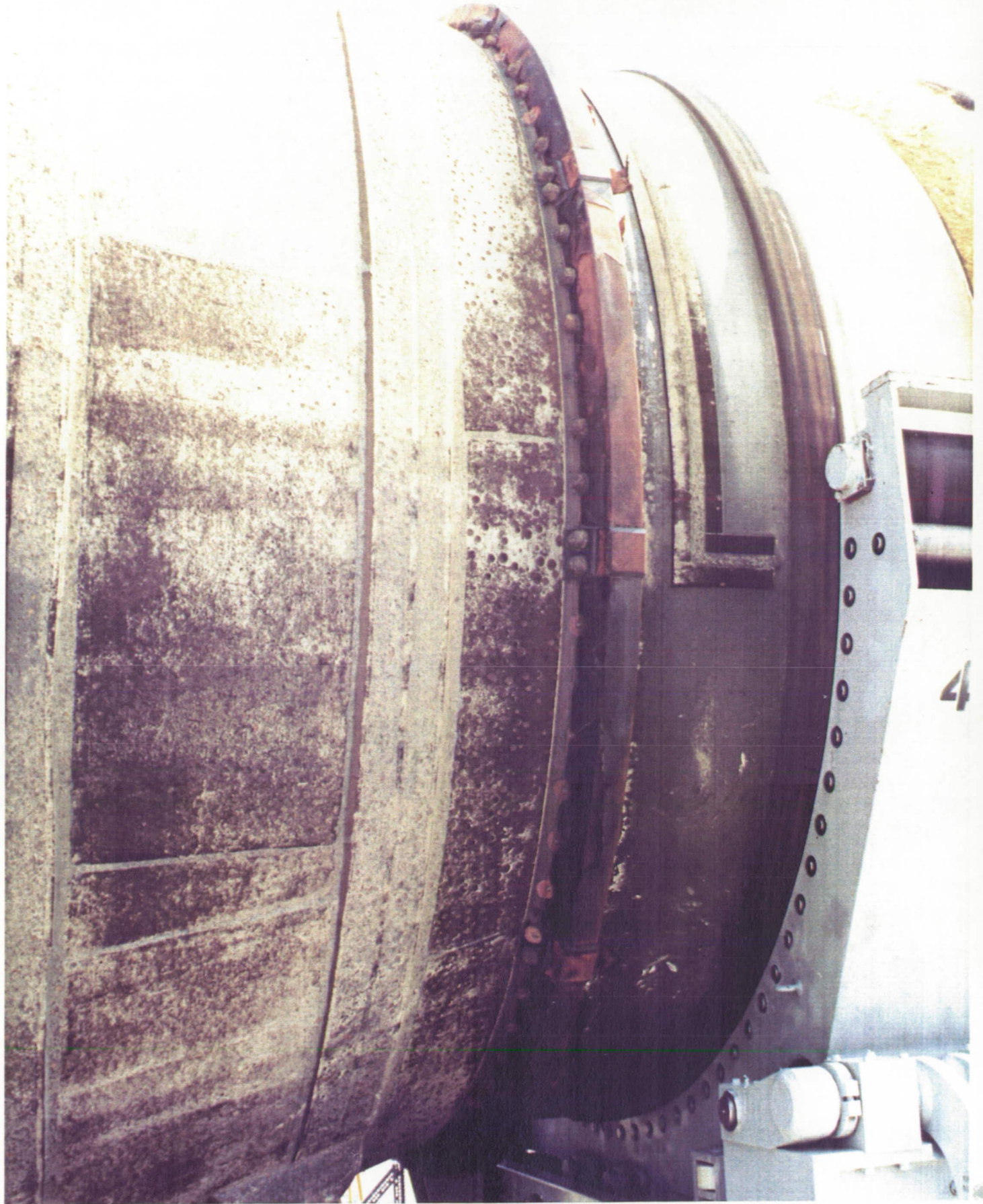
K5NA protective domes were lost from bolt heads on the aft side of the phenolic kick ring prior to water impact and exhibited a sooted substrate.
