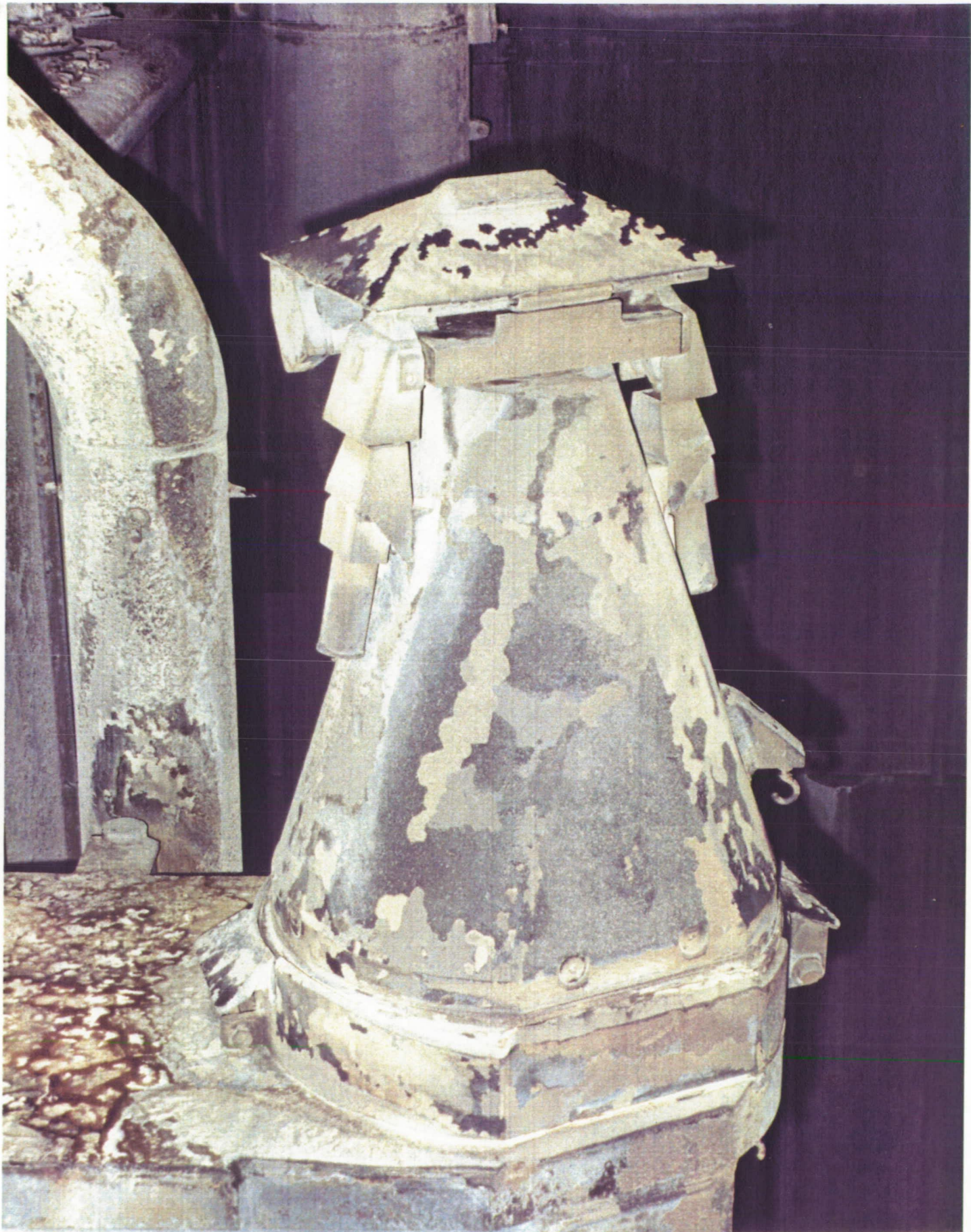
North HDP blast covers were in the closed position and exhibited typical SRB plume erosion effects
