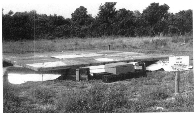
Receiving Flat-Plate Antennas
