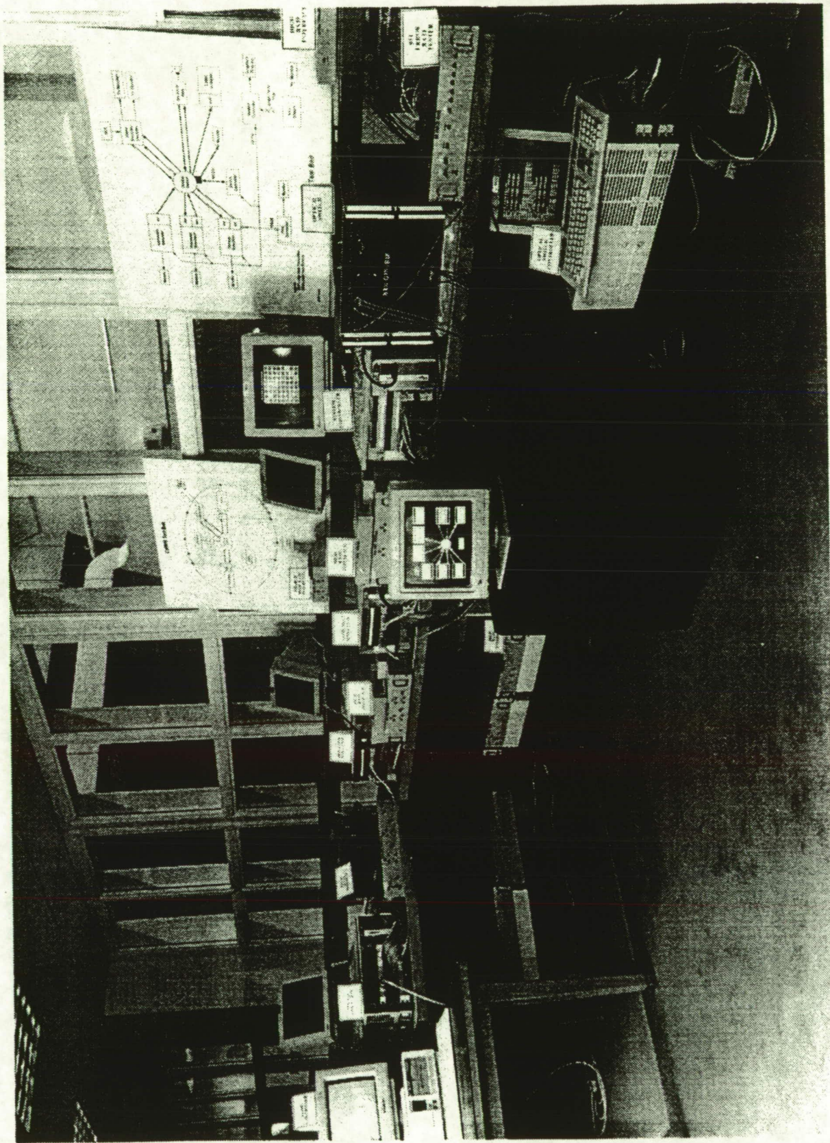
Figure 1-3. Photograph of CHRPS initial Test Bed configuration.
