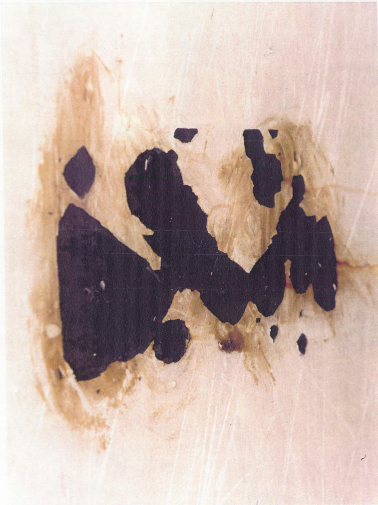
Several areas on the SRM segment cases exhibited missing paint and exposed metal substrate.
