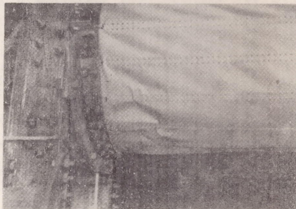
Figure 32.- Failure of full shell with closed-hat channels under bending with transverse load (outside view).
