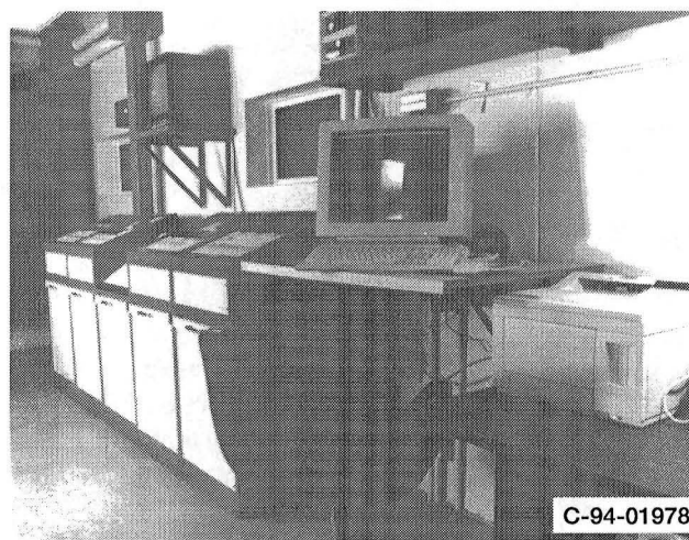
Figure 7.—Control room consoles.
