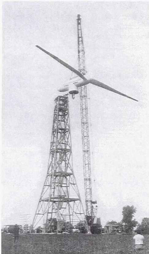
Figure 2. Final assembly of the 100-kW Mod-0 HAWT test bed in 1975. It was located at the NASA-Lewis Plum Brook Test Station near Sandusky, Ohio.
