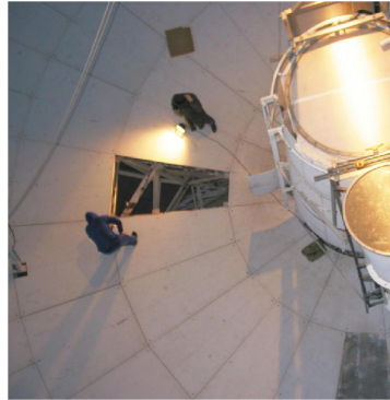
Figure 2. Night alignment of the 26-m antenna new surface panels; Cassegrain cone and 18 cm feed horn seen from top; theodolite reference target mounted beneath (removed) panel.
