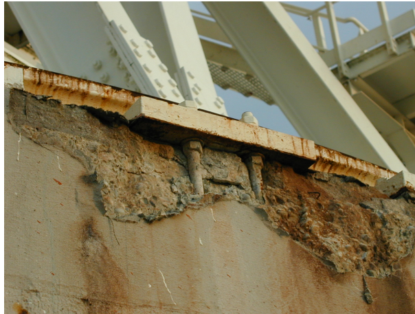
Figure 2. Rail at one of the damaged points (concrete was manually removed)
