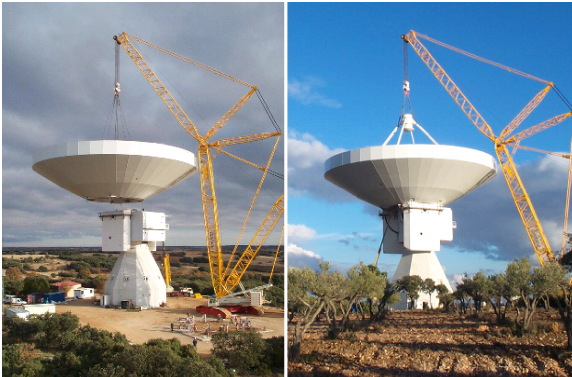
Figure 1. Erection of the new 40 meter radiotelescope of OAN at Yebes (Guadalajara, Spain).
