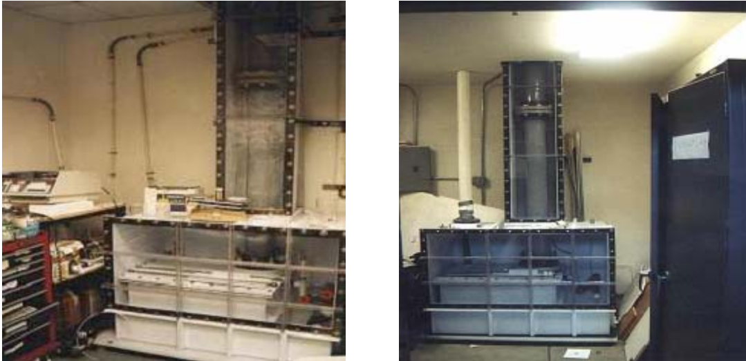
Figure 17. Inside (left) and outside (right) scrubber assembly including CM4 connections
