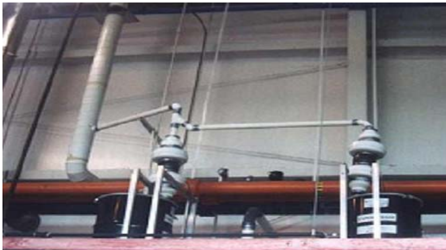
Figure 18. Drums containing activated carbon impregnated with KOH and exhaust fans assembly
