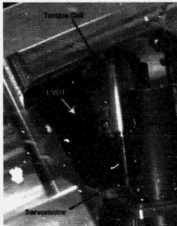
FIGURE 2-22. HOUSING FOR SERVOMOTOR, TORQUE CELL, AND LVDT (Photographed under the wing, near the trailing edge.)
