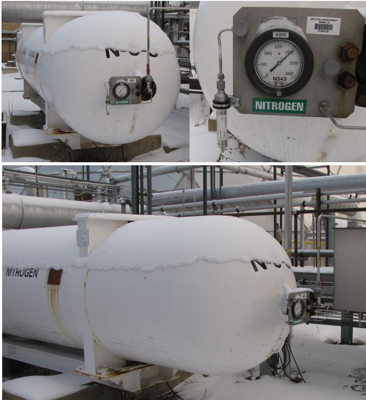
Figure 2.—Views of data logging transducer installation at Glenn Research Center, Cleveland, Ohio. Clockwise from top left: End view of the vessel and pressure indicating panel, close up of transducer mounting, profile view of vessel (only half of vessel is seen in this view).
