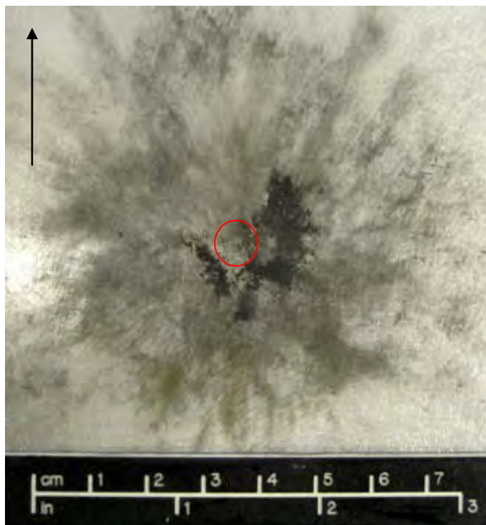
Figure 584 Close-up View of Damage to Front of Rear Wall (scale in 1cm increments / black arrow indicates flight path of projectile / cleaned)
