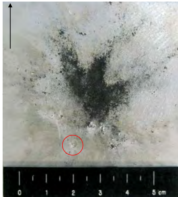
Figure 482 Close-up View of Damage to Front of Rear Wall (scale in 5mm increments / black arrow indicates flight path of projectile)
