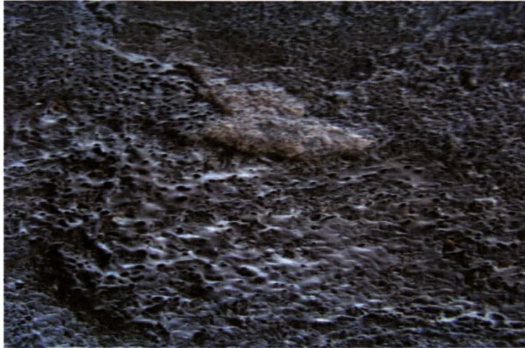
Figure 2. Possible melting of the refractory concrete surface
