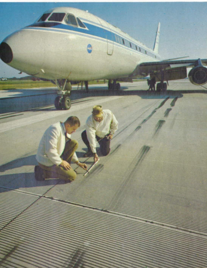
Transverse grooves on the airport runway provide a solution to "hydroplaning." In this test, the grooves were one-quarter of an inch deep and spaced about an inch apart.
