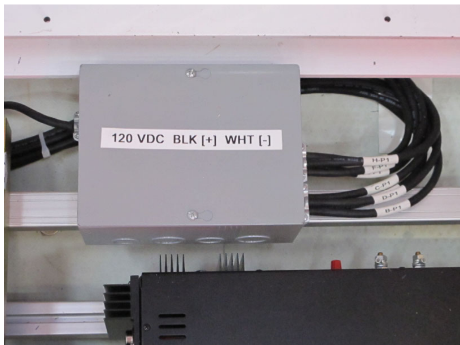
Figure 9.—120 VDC light power junction box.
