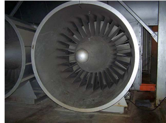
Axial Vane Fan at the Glenn Research Center's 10x10 Wind Tunnel
