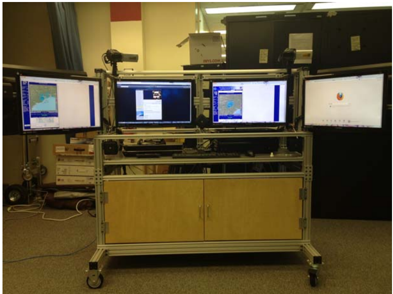
Figure 16: The MHW has been finished with the addition of the monitors, cameras, receiver, speakers, blu-ray players, desk, and cabinet doors.
