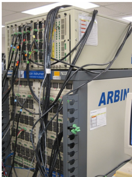
Figure 6.—Arbin battery test system.
