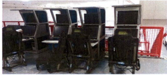
Figure 1. Table Four Computer Com Center. Each computer was equipped with dual monitors, a keyboard and a mouse. The Command Center took approximately 1 week to fully setup.
