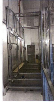
Figure 8. Don/Doff In this area the engineers will be putting on respirators and clean suits.
