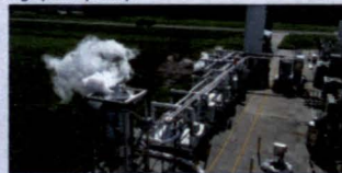
Propellant Transfer System
