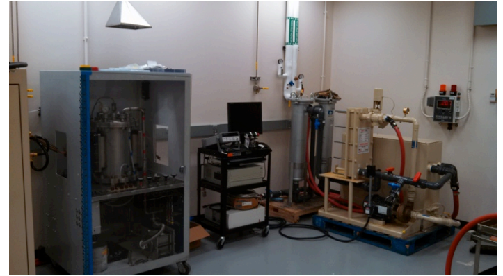
CFEET pumps and containment
