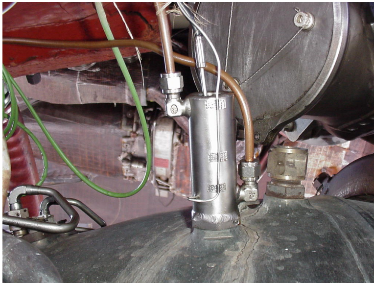
Installation at 337°, CCW, aft looking forward
