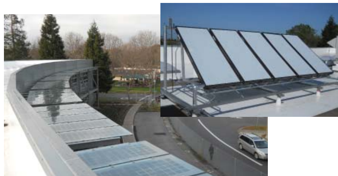
Solar panels on the new 'green building.'
