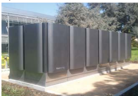
Fuel Cell near Building, 232
