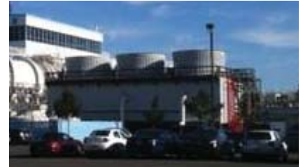
Ames Renovated Boiler System
