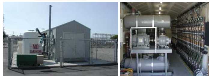
Exterior (Left) and interior (Right) views of the air Sparge System
