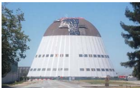
The shell of Hangar 1 being removed, May 2011. For more information visit http://www.nasa.gov/centers/ames/home/2008/hangar_index.html
