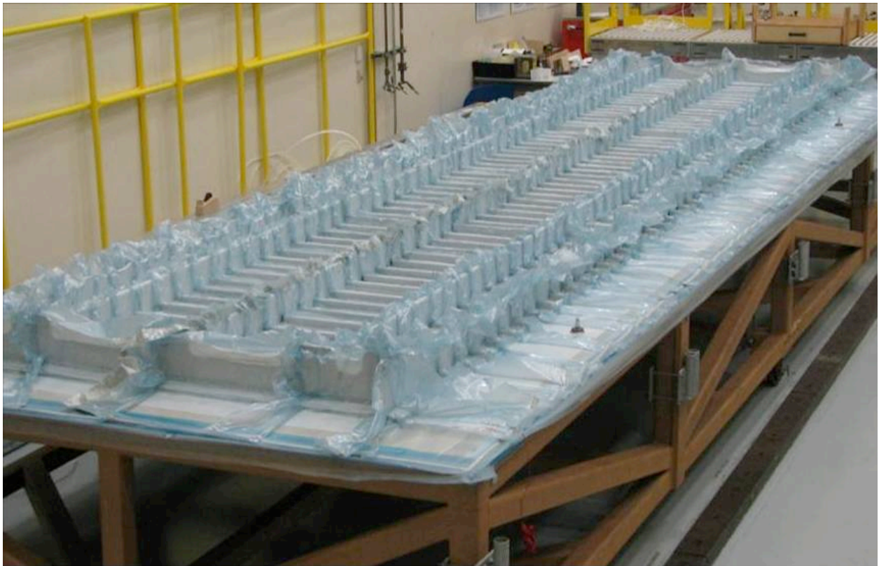
Figure 52. Bagged Crown Panel with IML-side Up and Repair Patches Taped to the OML
