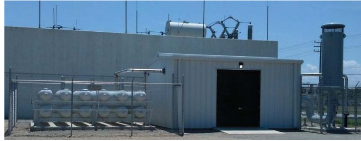
Figure 14. High Pressure Air Reducing Station
