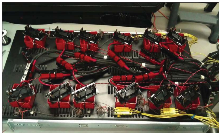
Fig. 4: Assembled 12-battery test bed rack
