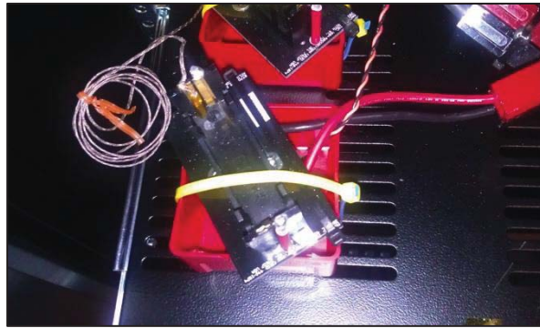
Fig. 3: Battery cell holder showing power, sense cables and isolated thermocouple wire
