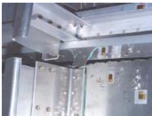
(b) Failed tear strap and frame
