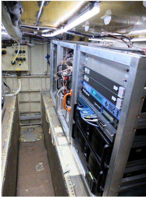
Figure 6.—Aircraft equipment racks.
