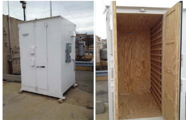
Figure 13—GRC advanced monopropellant storage locker.
