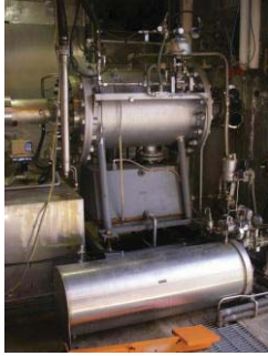
Figure 5. RCL-11 Water Cooling System with Two-Stage Dewatering Subsystem
