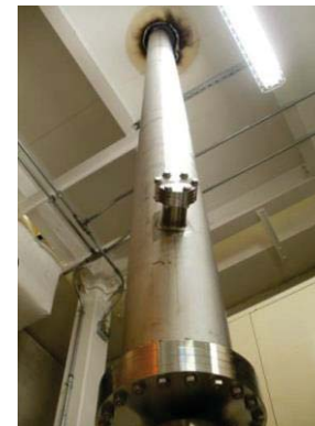
Cryogenic Container located at MSFC (below deck)
