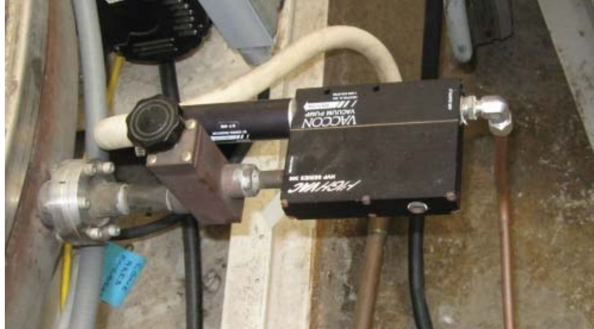
Figure 5.—The venturi pump on VF13.
