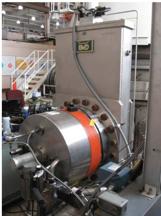
Figure 8.—The cryogenic pump on VF13.
