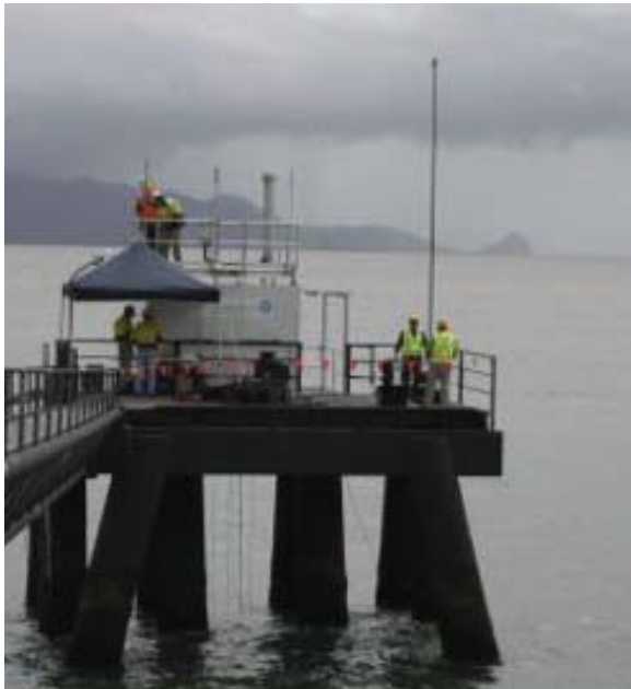
Fig. 10. Cable and instrument installation discussions on board the Lucinda Jetty Coastal Observatory (LJCO) off the coast of Lucinda, Australia.
