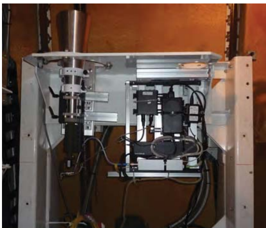
Fig. 4 Wideband (IGUANA) feed installed in the receiver room of Kashima 34m telescope.
