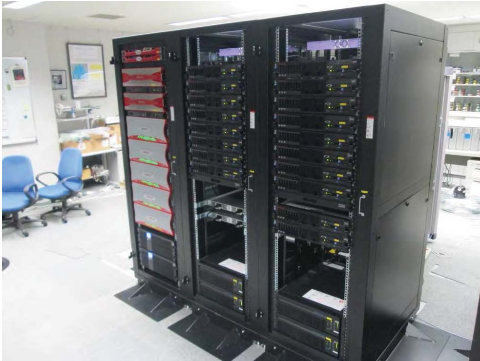
Fig. 2 New high performance servers and storage at the Tsukuba VLBI Correlator.
