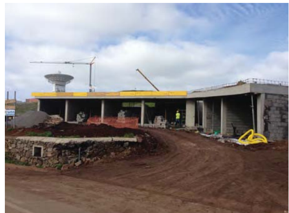
Fig. 4 Status of construction of the control and auxiliary buildings of the RAEGE station in Santa Maria.
