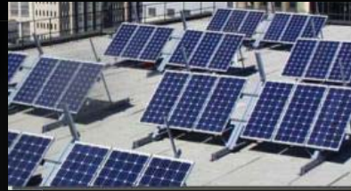
Rooftop PV Solar
