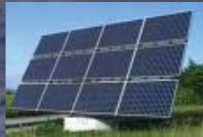
Ground PV Solar Array
